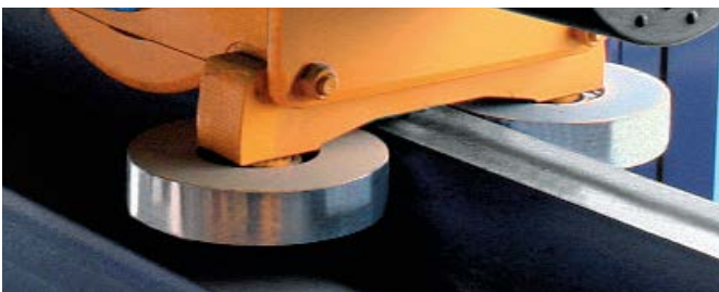
Guide rollers on the high level crane rail
